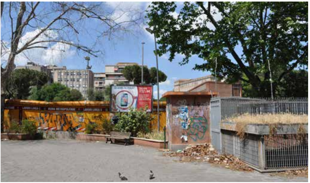
Fig.2 Metro Line C Construction in the Piazza Ipponio, photo by Madeleine Galvin.
